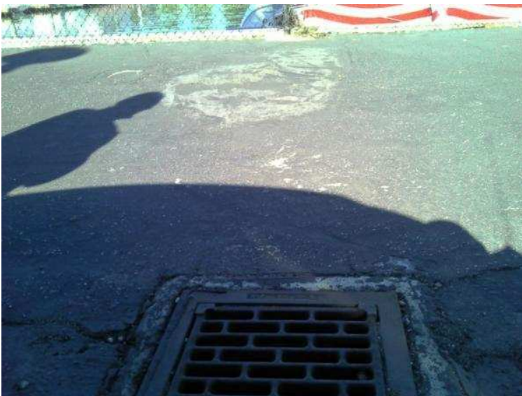
Figure 8. Catch Basin at The BoatYard
