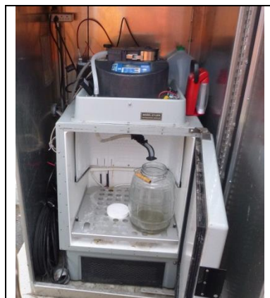
Figure B-3. ISSCO Type Automated Flow and Sampling Equipment
