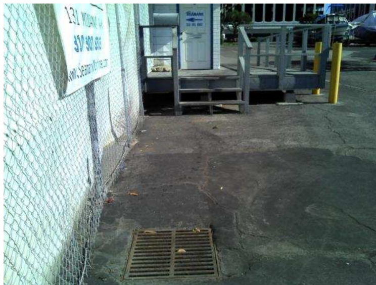
Figure 14. Example Catch Basin at Seamark
