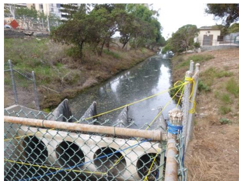
Material: Open channel upstream of four outfalls (inflow from 42-inch RCP) Tributary Area: 154.4 acres (8.3% MdR Watershed)
