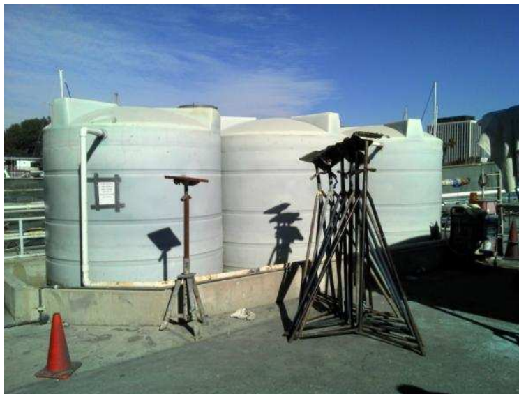
Figure 10. Settling Tanks at The BoatYard
