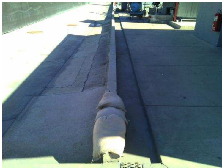
Figure 4. Flow Detention at Windward
